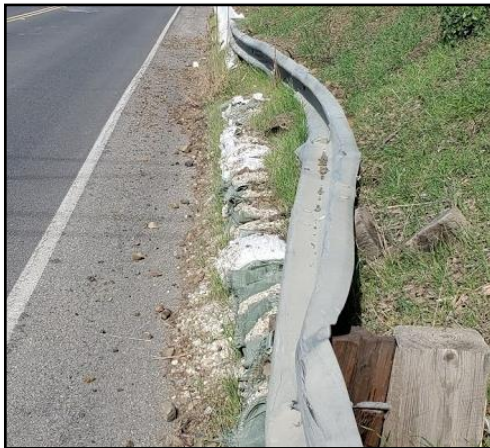
Damaged Guardrail and Narrow Shoulder
