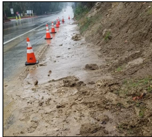
Erosion Prone Hillsides and Narrow Shoulder
