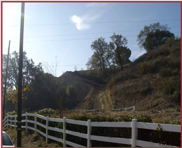
Unpermitted grading on hillside
